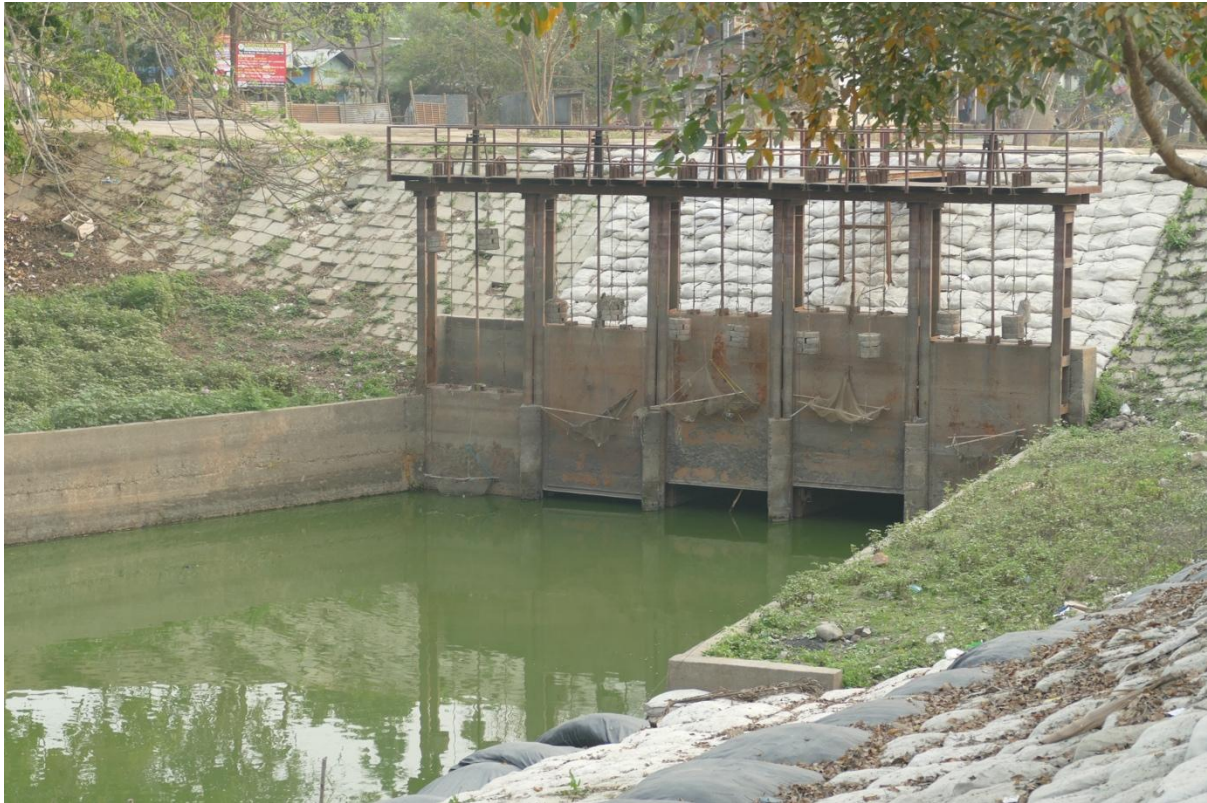
Photo 7: The sluice gate on the Khanajan rivulet which was constructed to reduce flooding in the area has become an impediment to the fish passage and movement between the Deepor Beel and the Brahmaputra River. (Photo in 2021)
